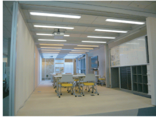
Fig. 9. Appearance of Intelligent Lighting System
