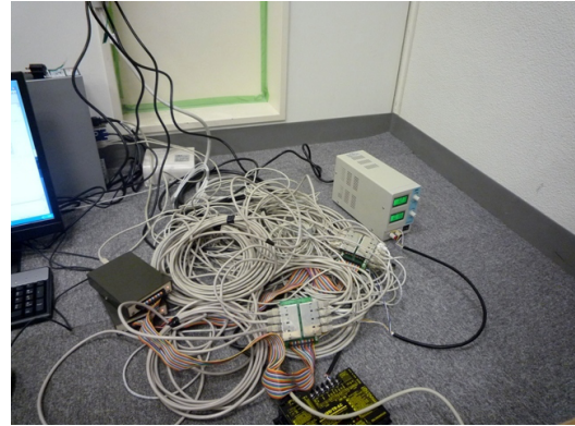
Fig. 4. Wiring status (Placed under the floor)
